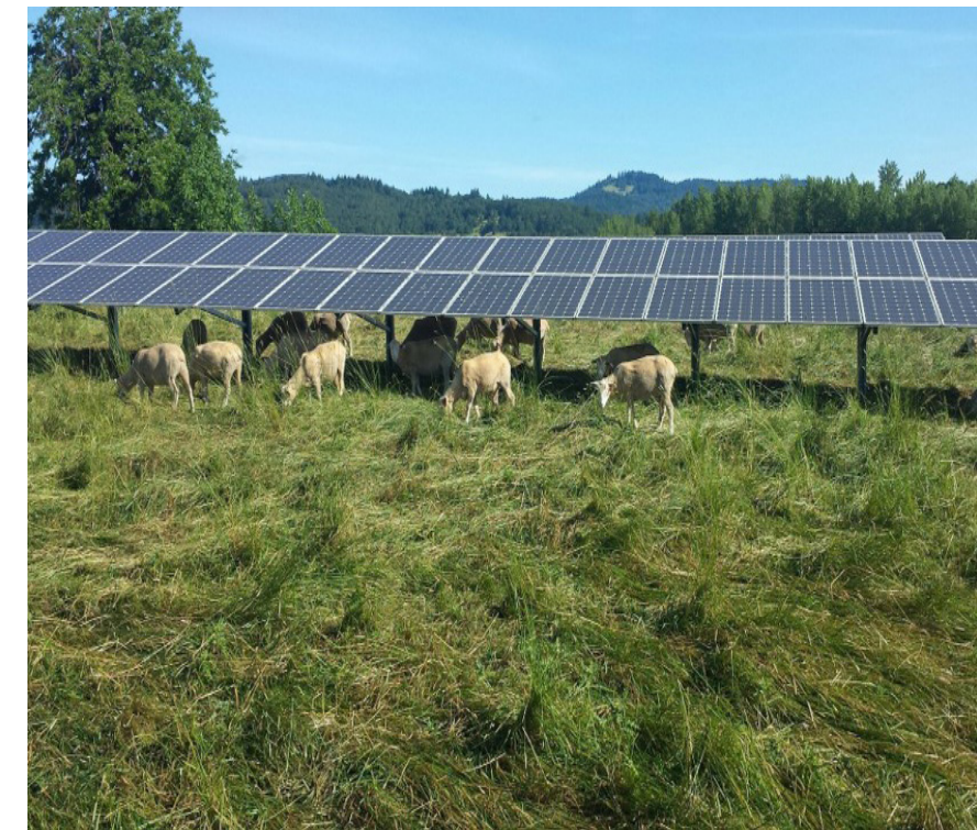
Crops grow while solar arrays create energy.
